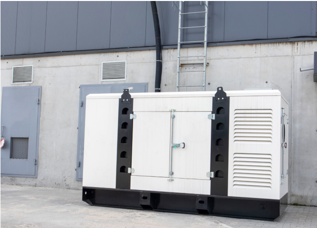
Coupling fitted between the engine and alternator.
